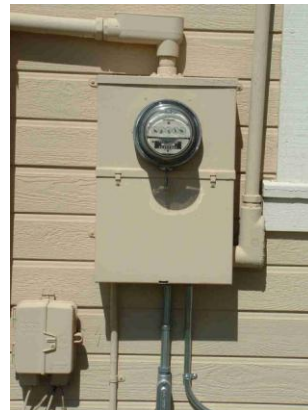
Outside: Circuit breakers for freezers #1 & #2 are located under the PG&E meter.
