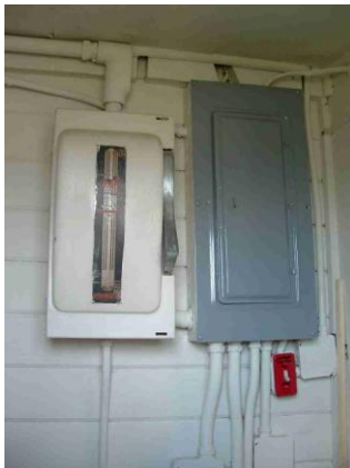
Inside the utility room: Grey box has circuit breakers for all heaters. Red box is circuit breaker for swamp cooler.
